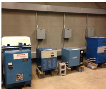
Electrical Vault Images by Delta Airport Consultants
