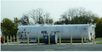
Above-Ground Fuel Storage Tanks Image by Delta Airport Consultants, Inc.
