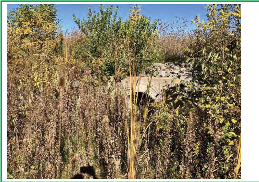
Photo 16: Stormwater culverts draining into Wetland B. Photo facing north.
